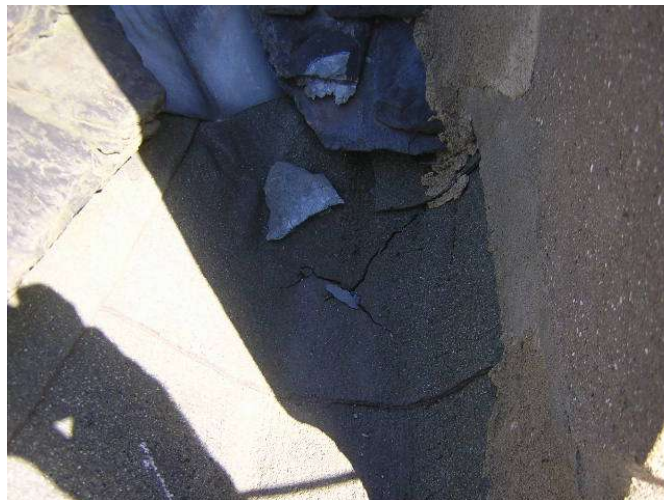
Defective Mineral Felt.
